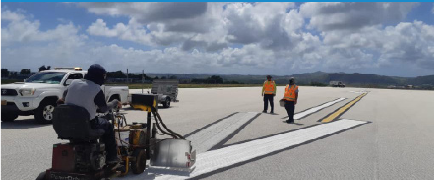
RUNWAY REFRESH. Personnel from the GIAA Properties & Facilities Building Section are seen refreshing critical runway surface markings in preparation for the Federal Aviation Administration (FAA) Flight Check, which is scheduled for March 3, 2023 and in anticipation of the re-opening of Runway 6L/24R, after a nearly two-year runway rehabilitation project.
